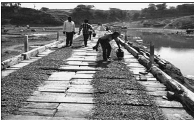
Photo 6 Preparation of Road Surface by Providing and Laying 20mm Thick Open Graded Premix Concrete with Liquid seal over Wooden Sleepers
