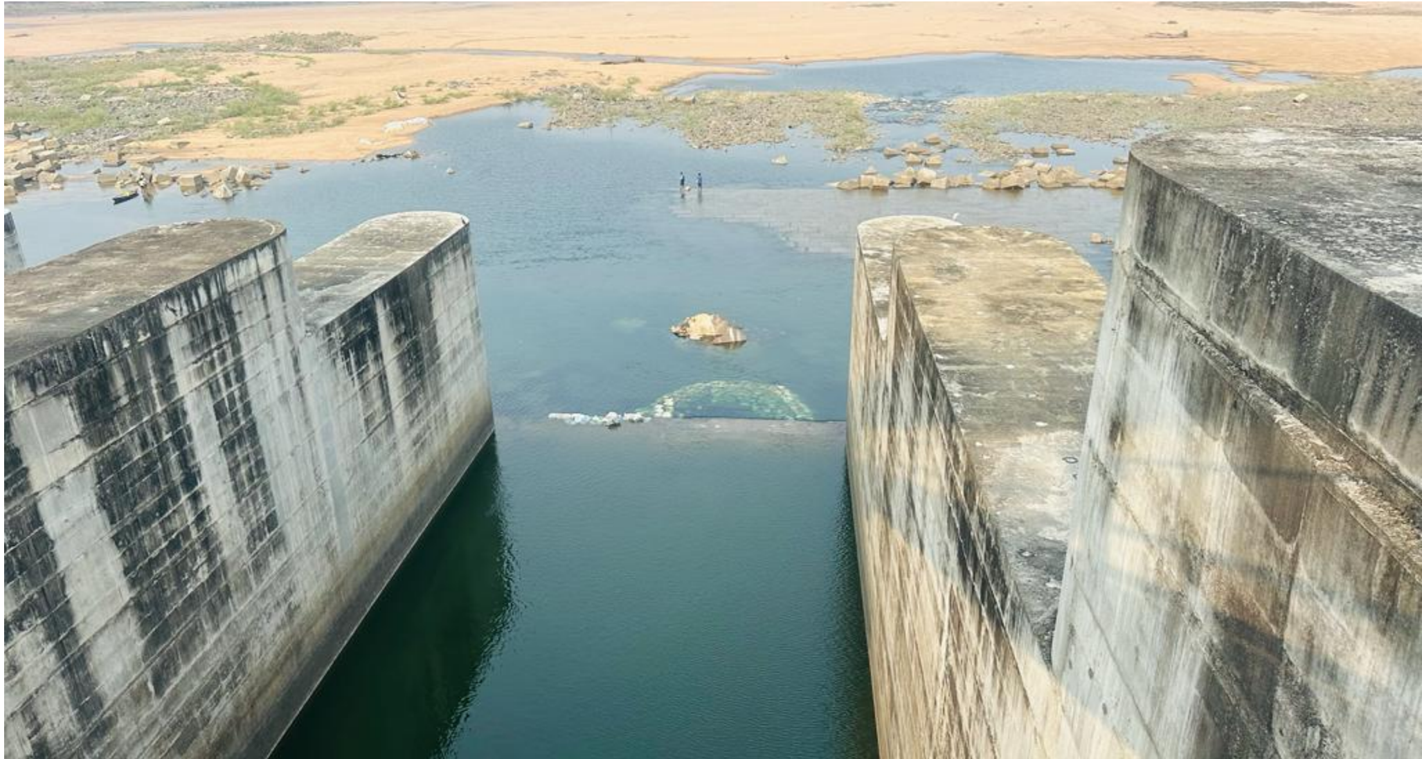
Visual-4: Visible seepage is observed in vent No-38 at downstream of Saraswathi Barrage
