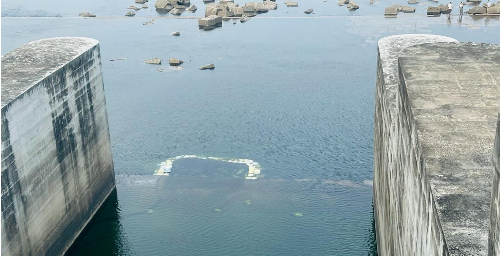
Visual-3: Visible seepage is observed in vent No-28 at downstream of Saraswathi Barrage
